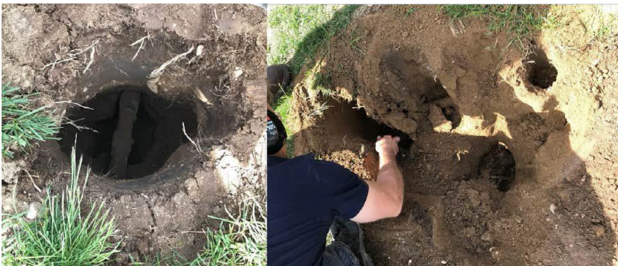
Figure 16 - Excavation results in the hard-compacted soil and removal of the soil from the surrounding area
